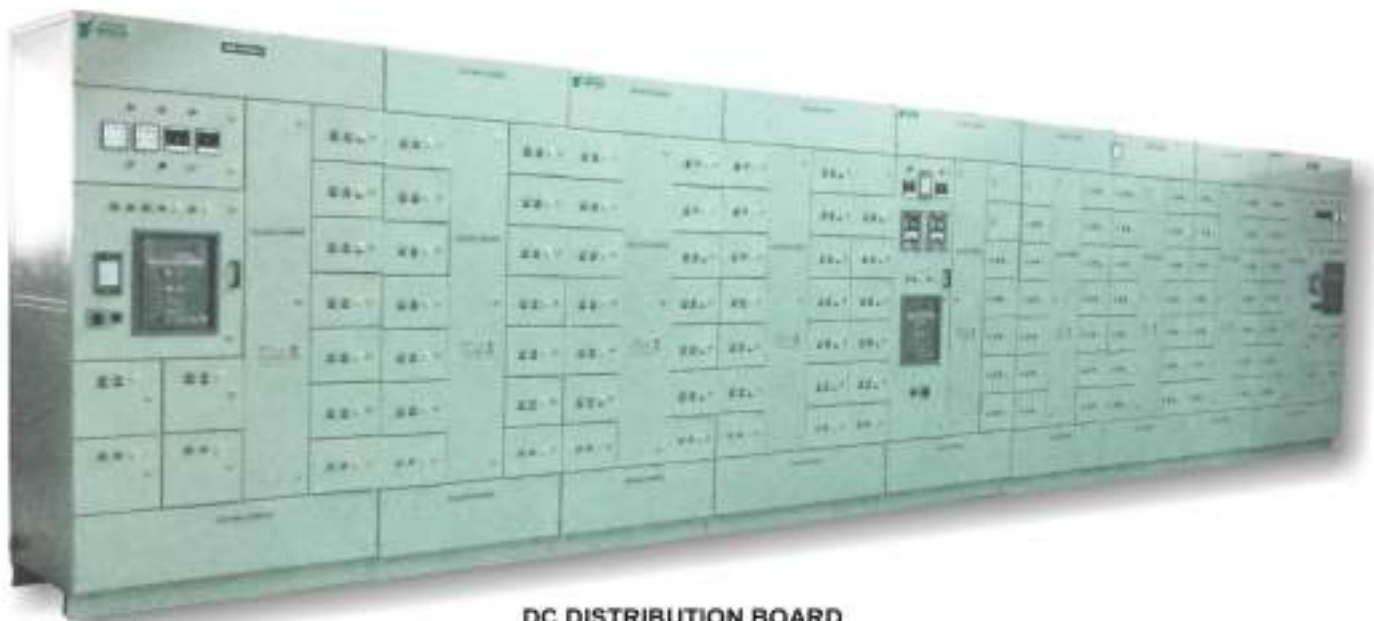
DC DISTRIBUTION BOARD
