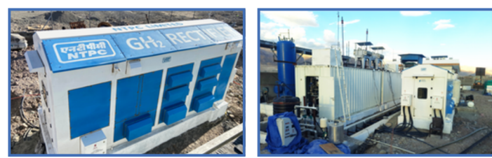
2x558kW Containerised Rectifiers - 3600A/ 155V for NTPC, Leh Green Hydrogen Mobility Pilot Project (Forced Air-Cooled; Outdoor Container Type)
