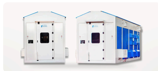
Two 558 kW containerised rectifiers, 3600 A / 155 V, forced air-cooled, outdoor container type, for a green hydrogen mobility pilot.
