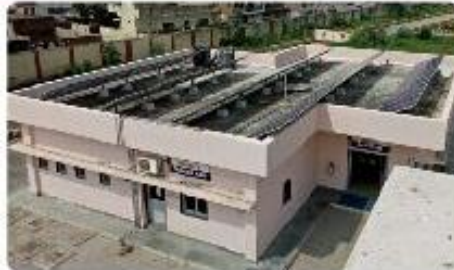
190kW PLANT AT IOCL, PUNJAB
