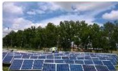
180kW KHUNTI CIVIL COURT
