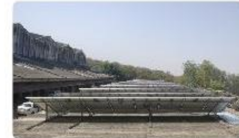
100kW KUMAR COLD STORAGE, LKO
